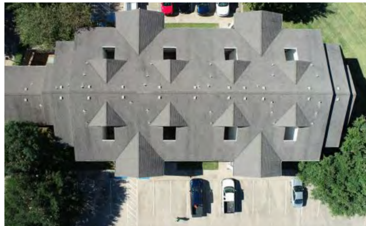
Blinn College Park Apartments Building #5, Aerial photography utilized for roof condition assessment.
